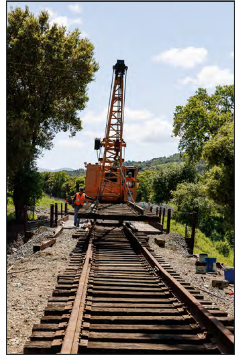
Chris Hauf photograph Rick Cory guiding track panel and Steve Barkkarie operating Burro crane over Happy Valley Road Bridge.
