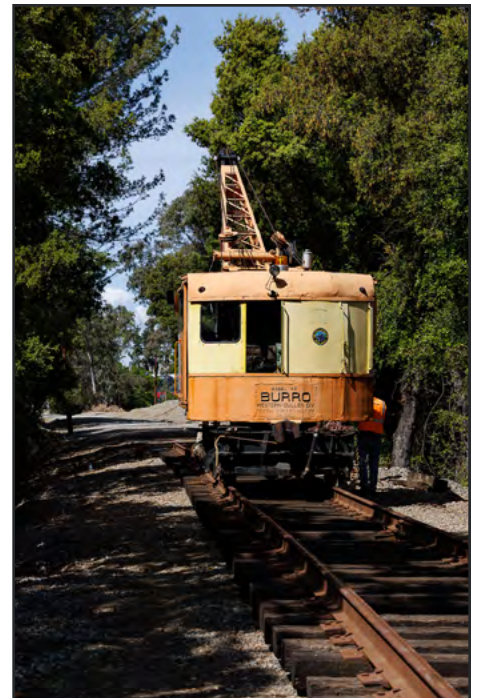
Chris Hauf photograph First piece of MOW equipment on track east of Happy Valley Road Bridge.
