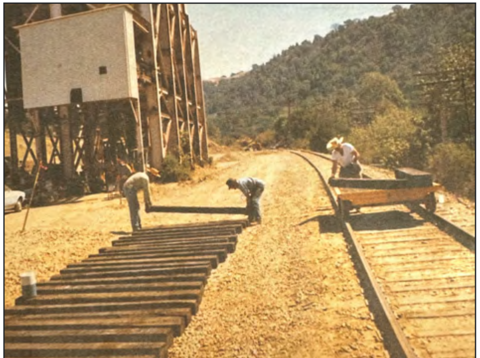
Track crew still extending siding at Brightside. Mark Whitman graded area for laying ties.
