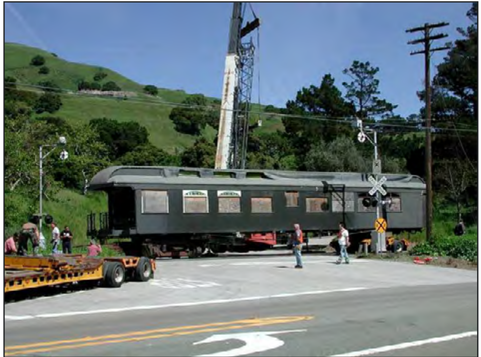
The crane setup before rolling the front truck under. The two visible stained glass windows were stacked by the author, the remaining 15 windows were crafted by volunteer Linda Schulz.
