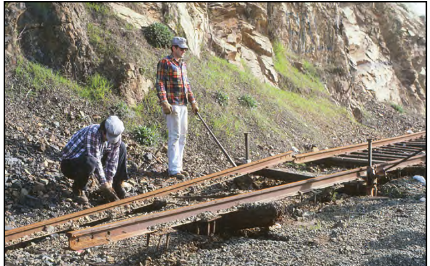
Mike McQuaid photograph Tim Flippo (standing), along with unidentified Castro Point Railway (CPRy) volunteer, using track jacks to remove rail from CPRy's location by the Richmond-San Rafael Bridge for use in Niles Canyon to protect ties left behind by Southern Pacific prior to CPRy's move there in 1986.
