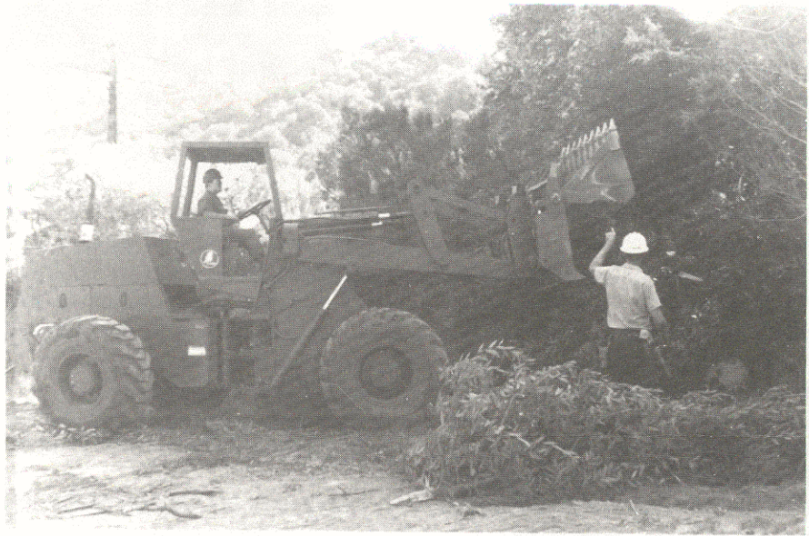
Craig Wilson directs a Seabee with hand signals as they clear out tree branches.
