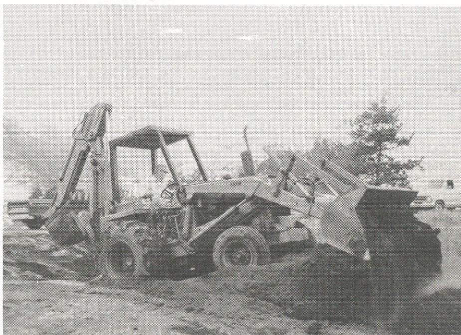
Frank Presley does roadwork with the PLA's Case 580B backhoe. The PLA will need the help of its members to finance this important acquisition. (See accompanying story.)
